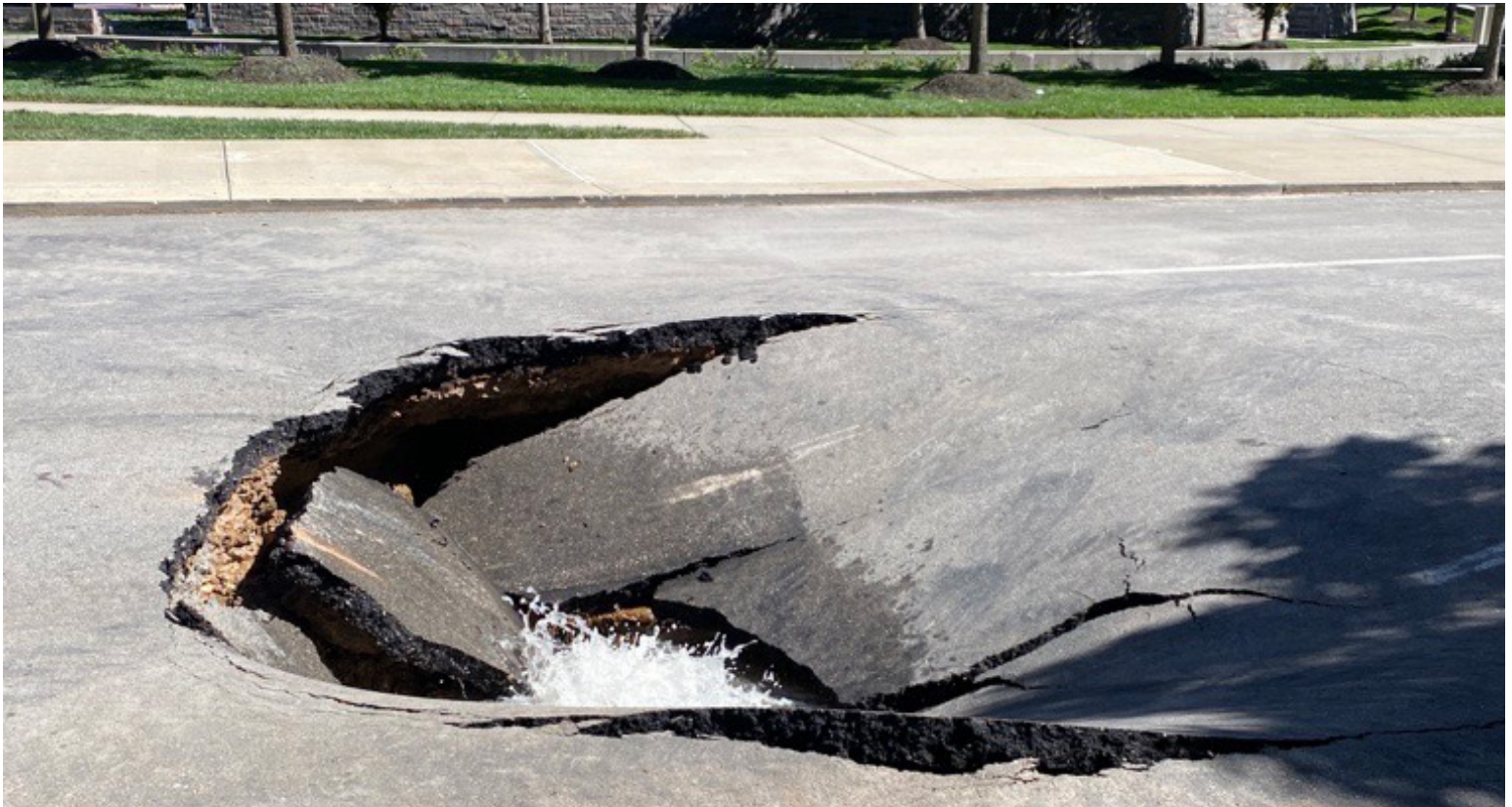
This water main break at 12th and Locust is why it is so important to invest in Kansas City's infrastructure. While repairing the water main break, crews discovered a collapsed combination sewer main.
