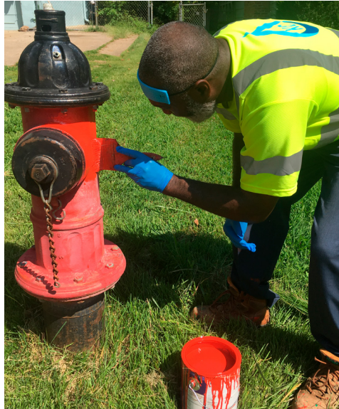
There are approximately 25,000 fire hydrants in Kansas City. Our goal is to repaint 5,000 hydrants a year.
