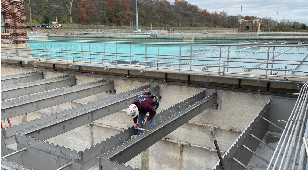
New, stainless steel weirs installed at the Water Treatment Plant will enable higher capacity flow of water being treated for taps and faucets of customers citywide.
