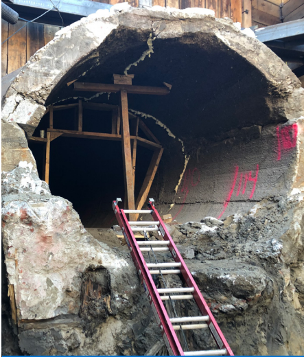
Rock and trash may accumulate in large diameter sewers, reducing or blocked wastewater flow that diminishes sewer system efficiency.
