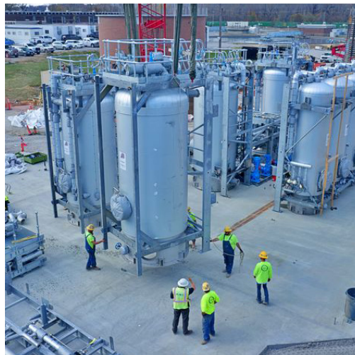
Thermal hydrolysis process equipment delivered to KC Water this fall will pressure cook human waste into reusable materials.
